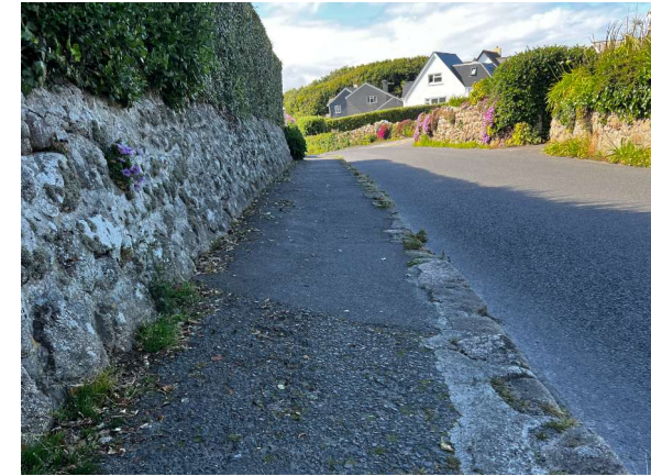
Footways are in poor repair and their kerbs are a fall hazard
