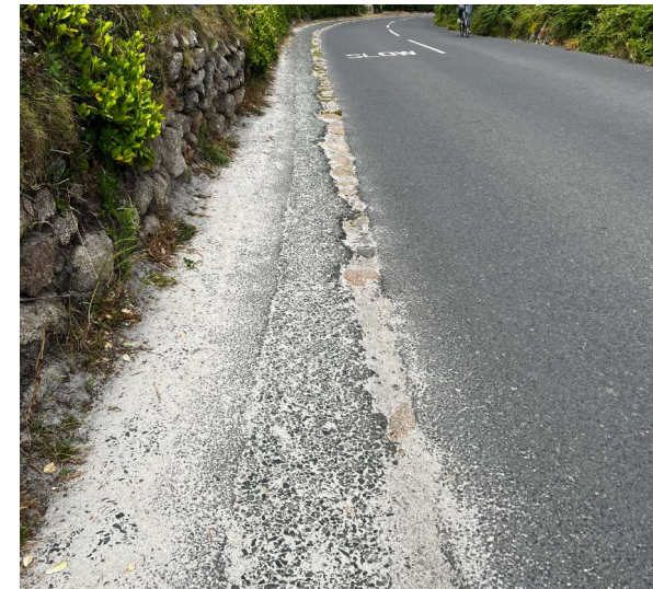
Poor quality narrow footway on route where traffic exceeds 20mph
