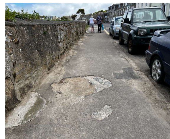
Footways across the island are generally in a poor state of repair.
