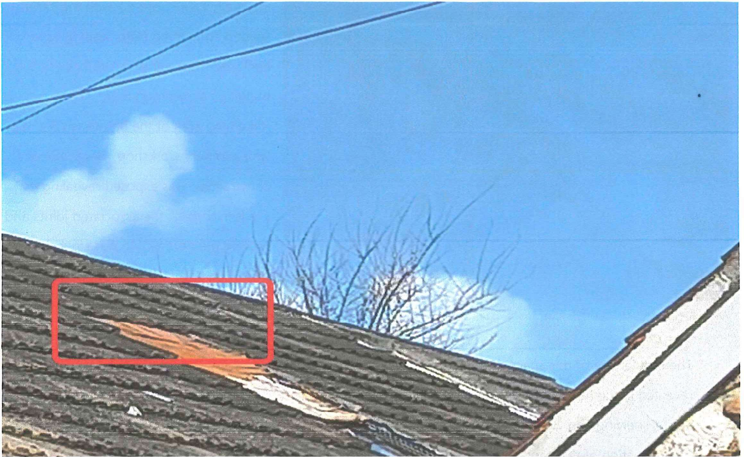
Photo 2. Gap between underlying sarking and roof tiles
