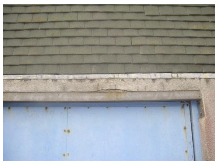
Failure of vertical tile hanging
