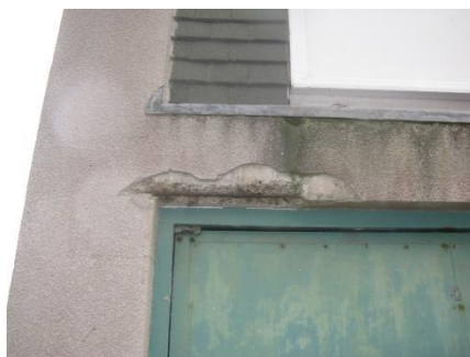
Corroded Reinforcement and spalled concrete to opening reveal
