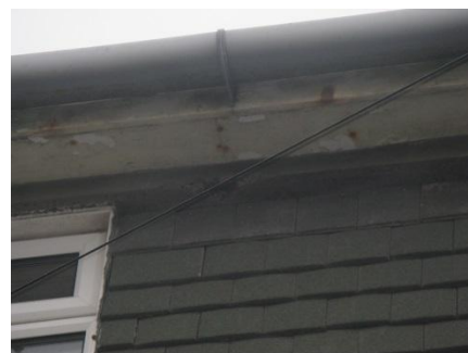
Poor condition of fascias and soffits.
