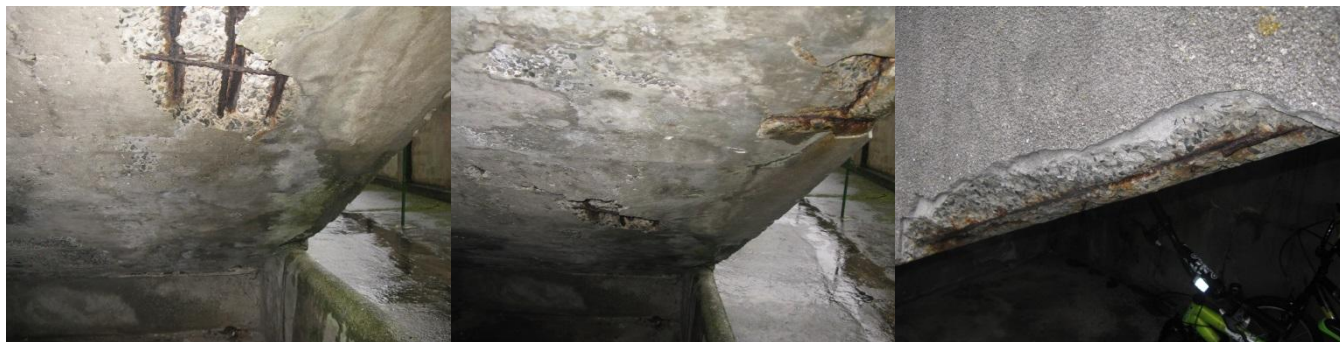
Corroded Reinforcement and spalled concrete to stairs
