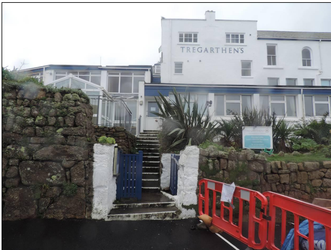
7. View to south side of east elevation. New entrance tower to be formed here.
