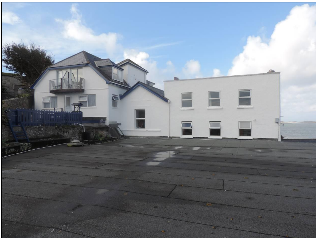
12. View of south elevation from south. Part of structure below to be removed.
