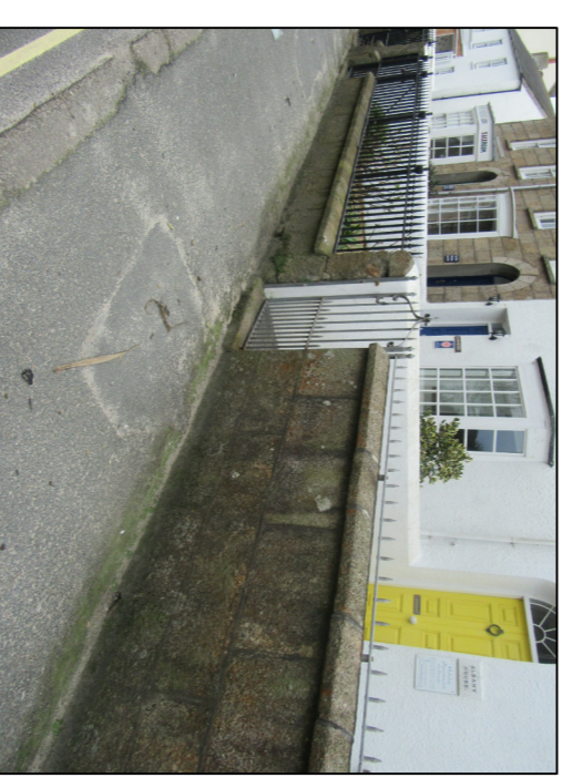
Replace wall railings and gate to match the neighbouring property
