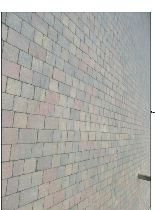
aving to all hardstanding areas to the rear of the building to match the above
