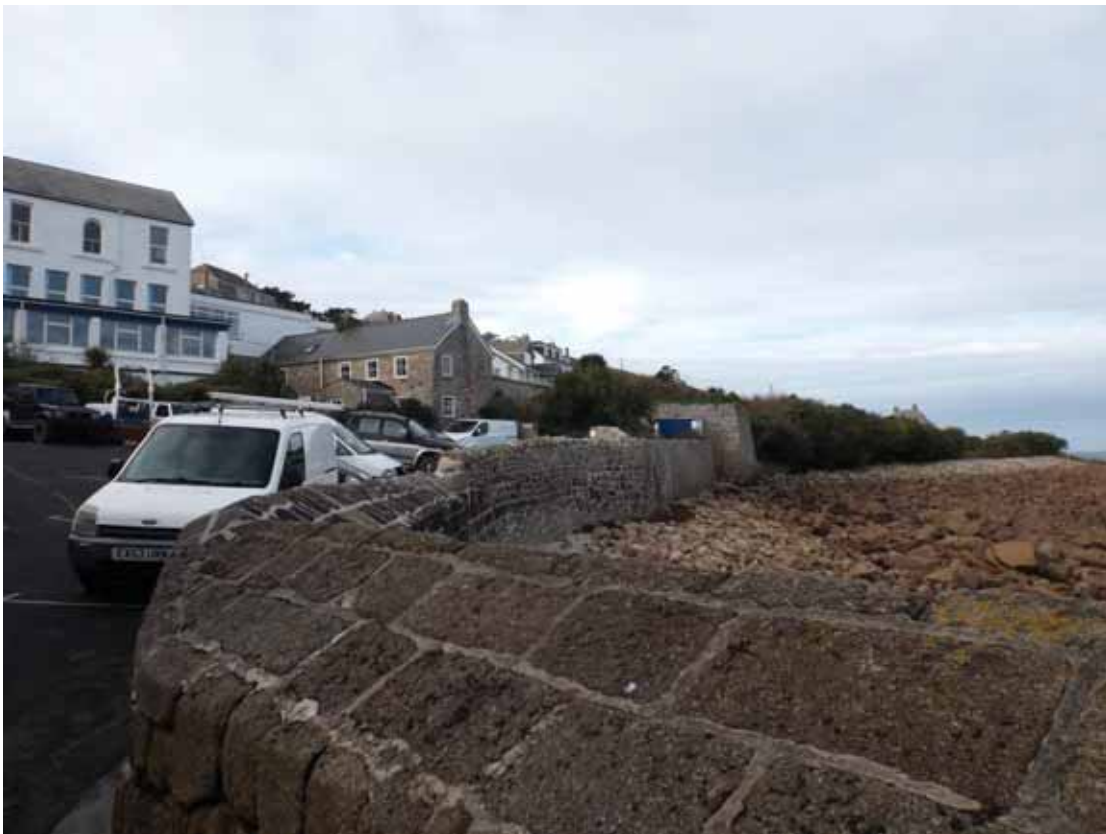
Plate 6: Detail of the sea wall, illustrating the height difference between sea-level and the main hotel buildings.
