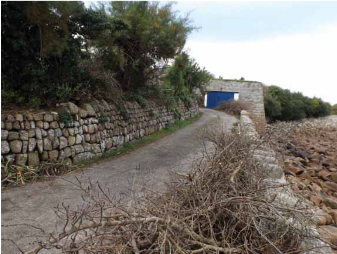
Plate 7: Detail of the sea wall and the garden retaining wall, at the northern end of the study site.
