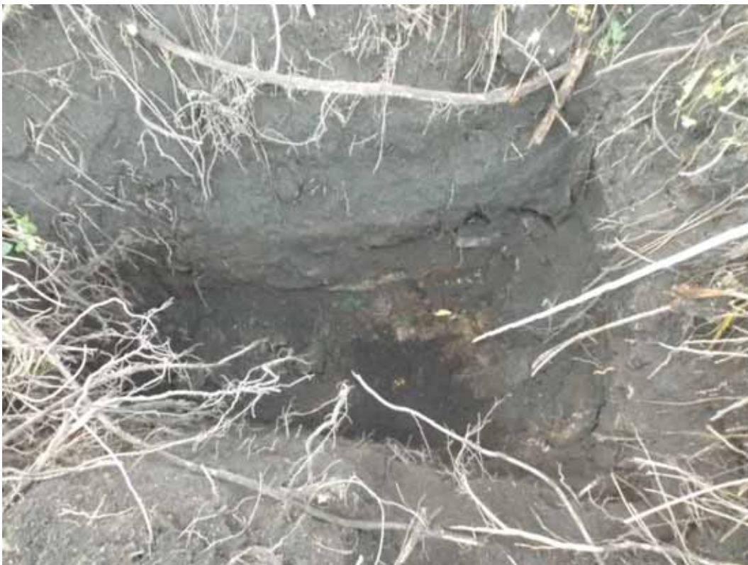
Plate 12: Geotechnical test-pit at north-east end of garden area. There is a single homogenous layer of dark garden soil lying above the ram, the weathered top of the underlying granite.
