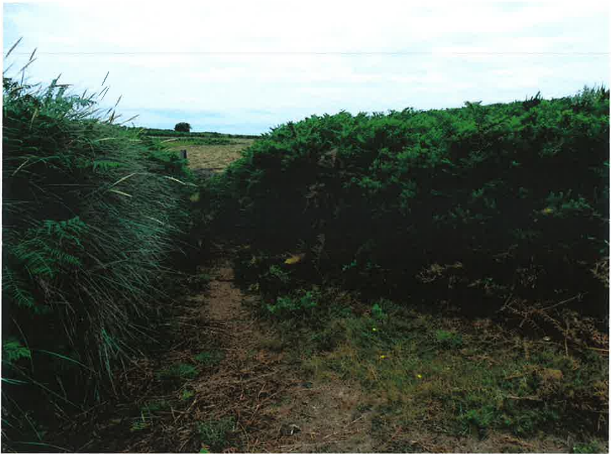
This picture looks 90 degrees left of the previous view and shows the direction to be taken by the pipe running to the soak away for the septic tank.
