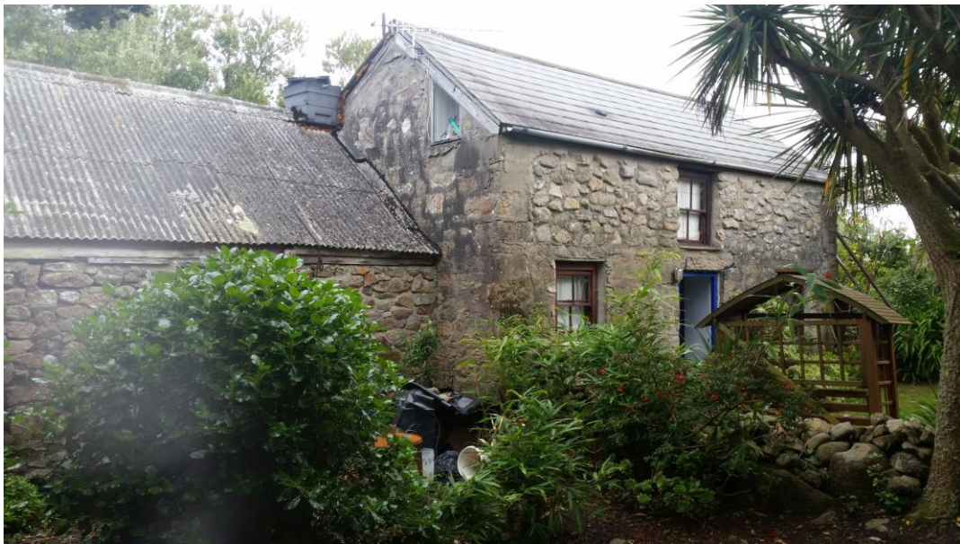
Fig. 5: South elevation of the Boatshed, to feature Solar panels under aluminium roof sheeting
