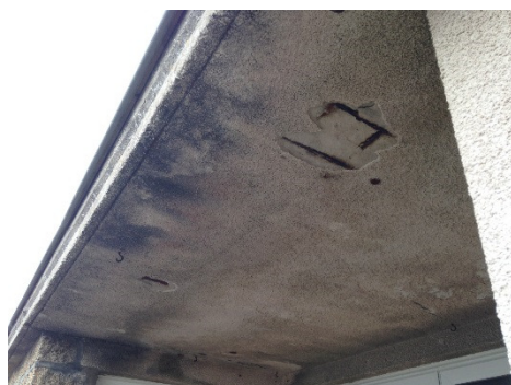
Reinforced concrete failure
