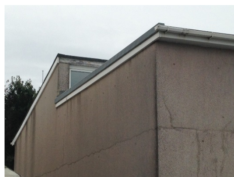
High level render failure
