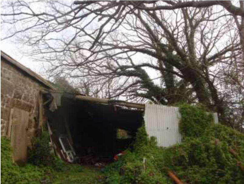
Fig 1.4 Large over-mature unbalanced Elms growing over building (not on Holy Vale site)
