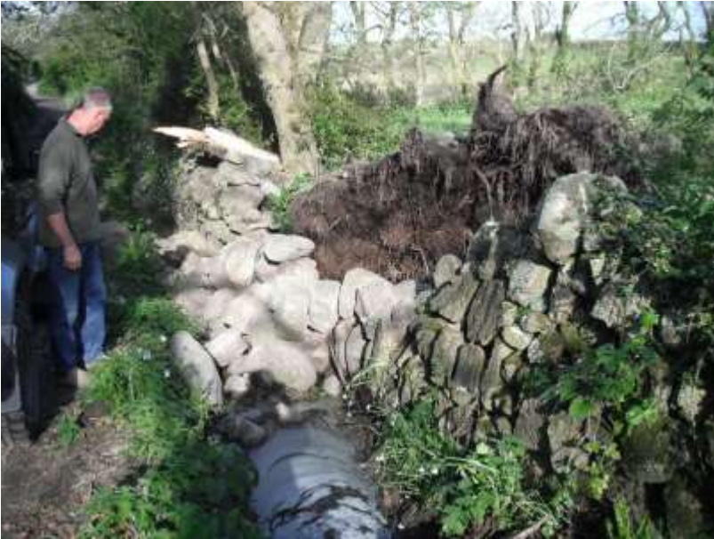
Fig 1.3 Mature Wind blown Elm with root ball damaging wall and run of water course (not on Holy Vale site)
