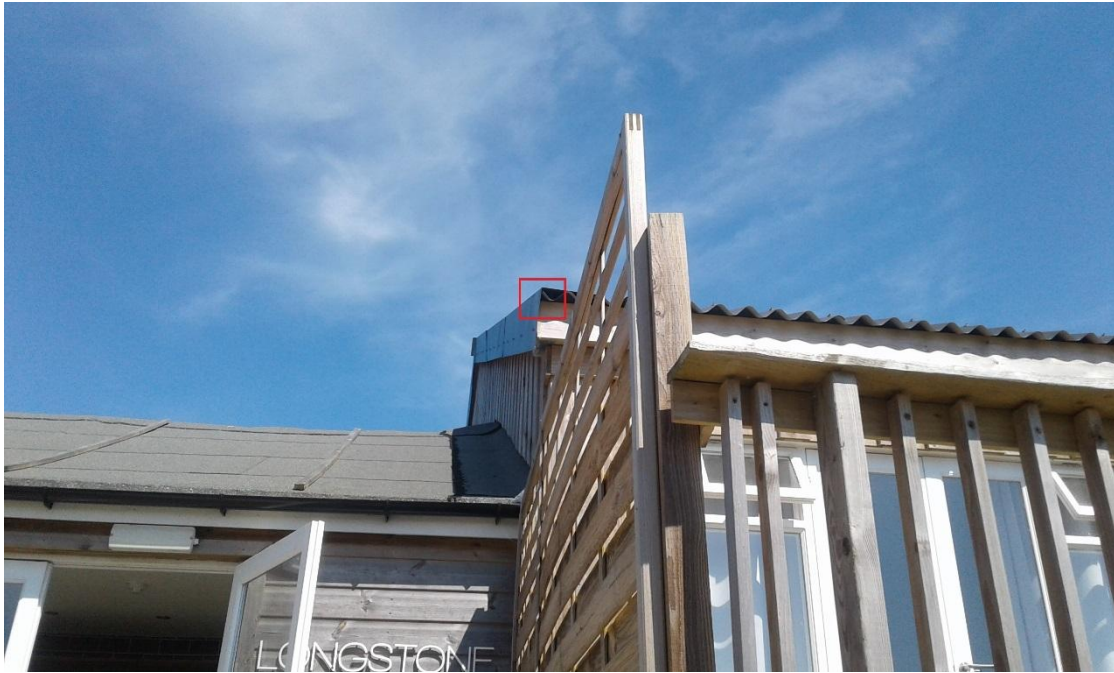
Photo 8. South west corner – void created where the barge flashing fits over the roofing sheet.
