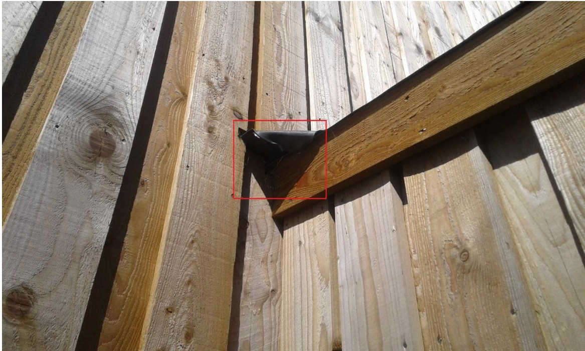
Photo 6. Porch on east aspect aspect – gap under lead flashing.
