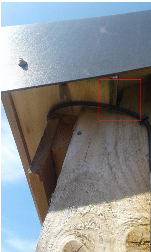
Photo 7. South east corner – gap at the top of timber.
