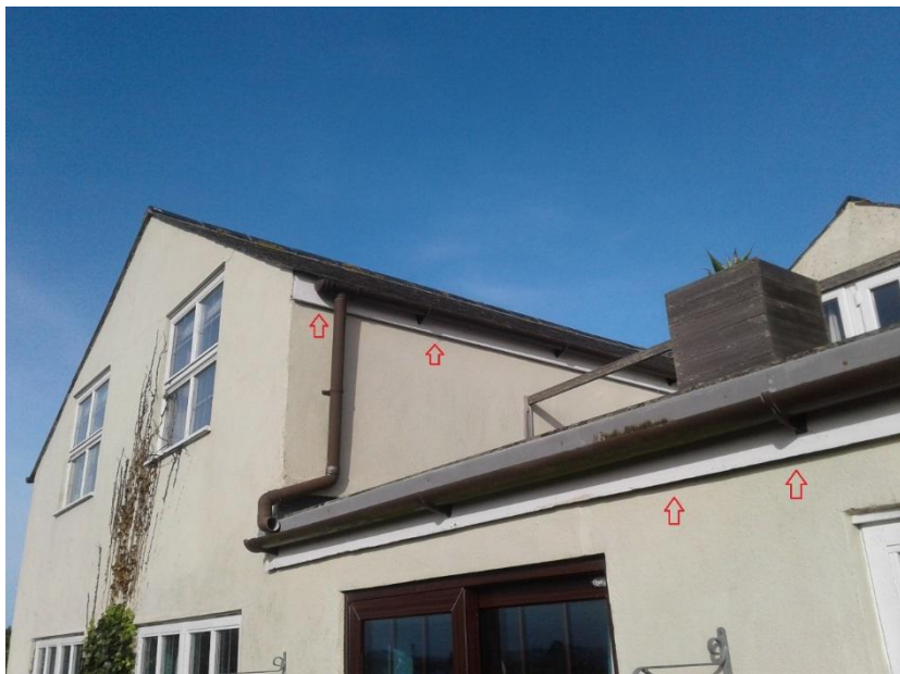
Photo 9 - Gaps behind the length of the soffit boards.
