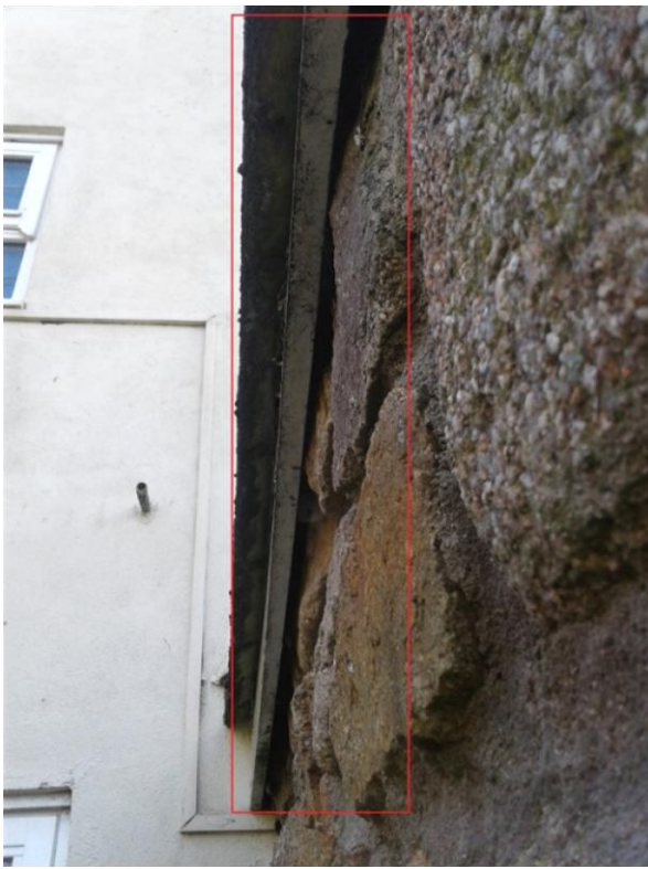
Photo 5 - Gapping behind the soffit on the porch.
