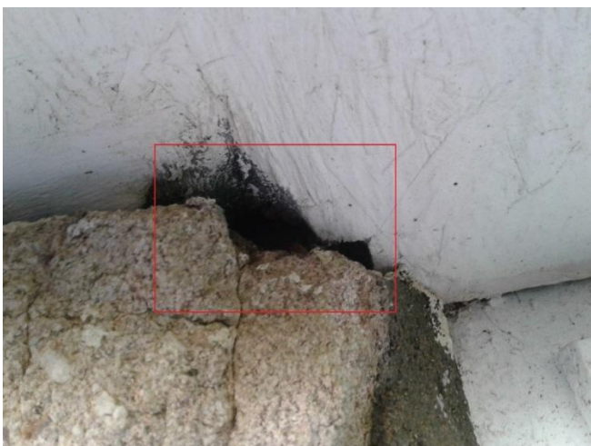
Photo 14 - Gap in soffit above granite.
