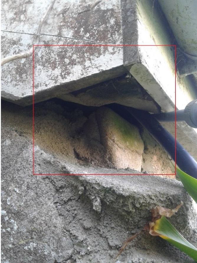
Photo 16 - Cavity behind the fascia boards.
