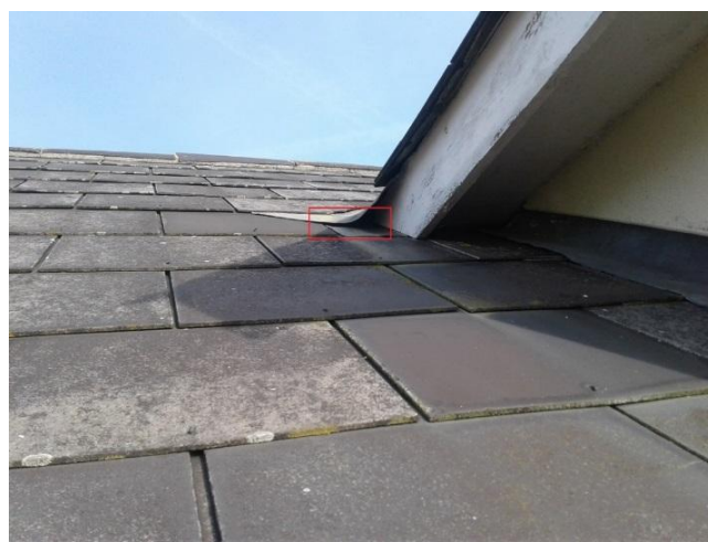
Photo 11 - Gap under flashing of the west dormer.
