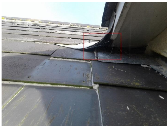
Photo 12 - Gap under flashing of the east dormer.
