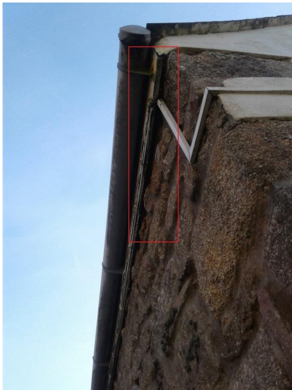
Photo 7 - Gaps behind the soffit.
