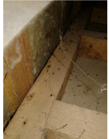
Photo 21 – Droppings on beam.
