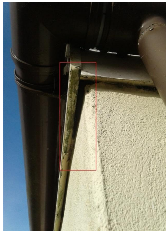
Photo 8 - Gap behind soffits.
