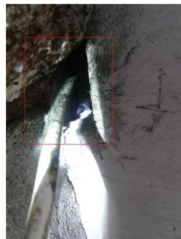
Photo 15 - Gap in soffit.
