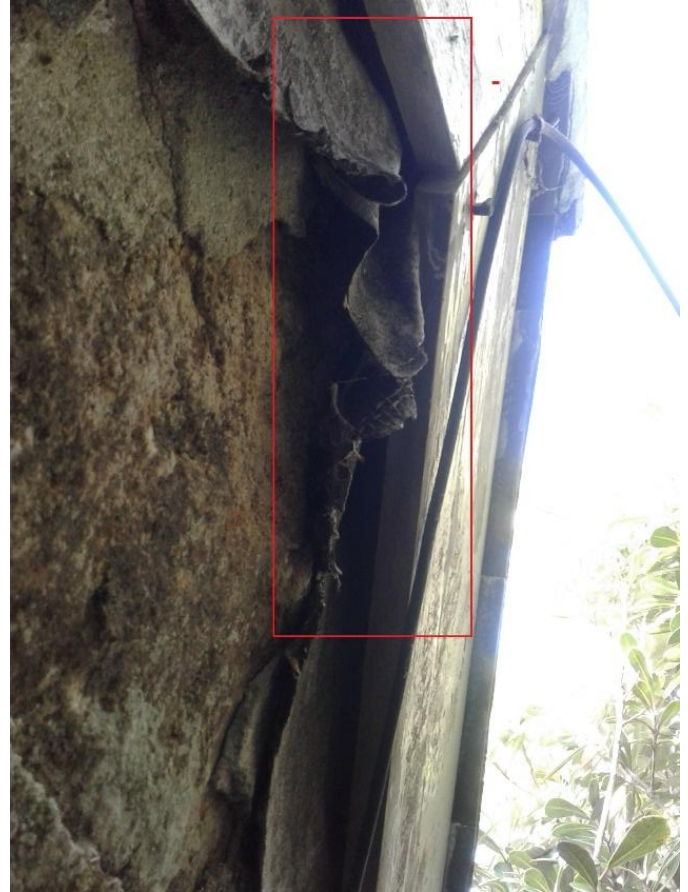
Photo 17 - Gaping between the bargeboard and the granite.
