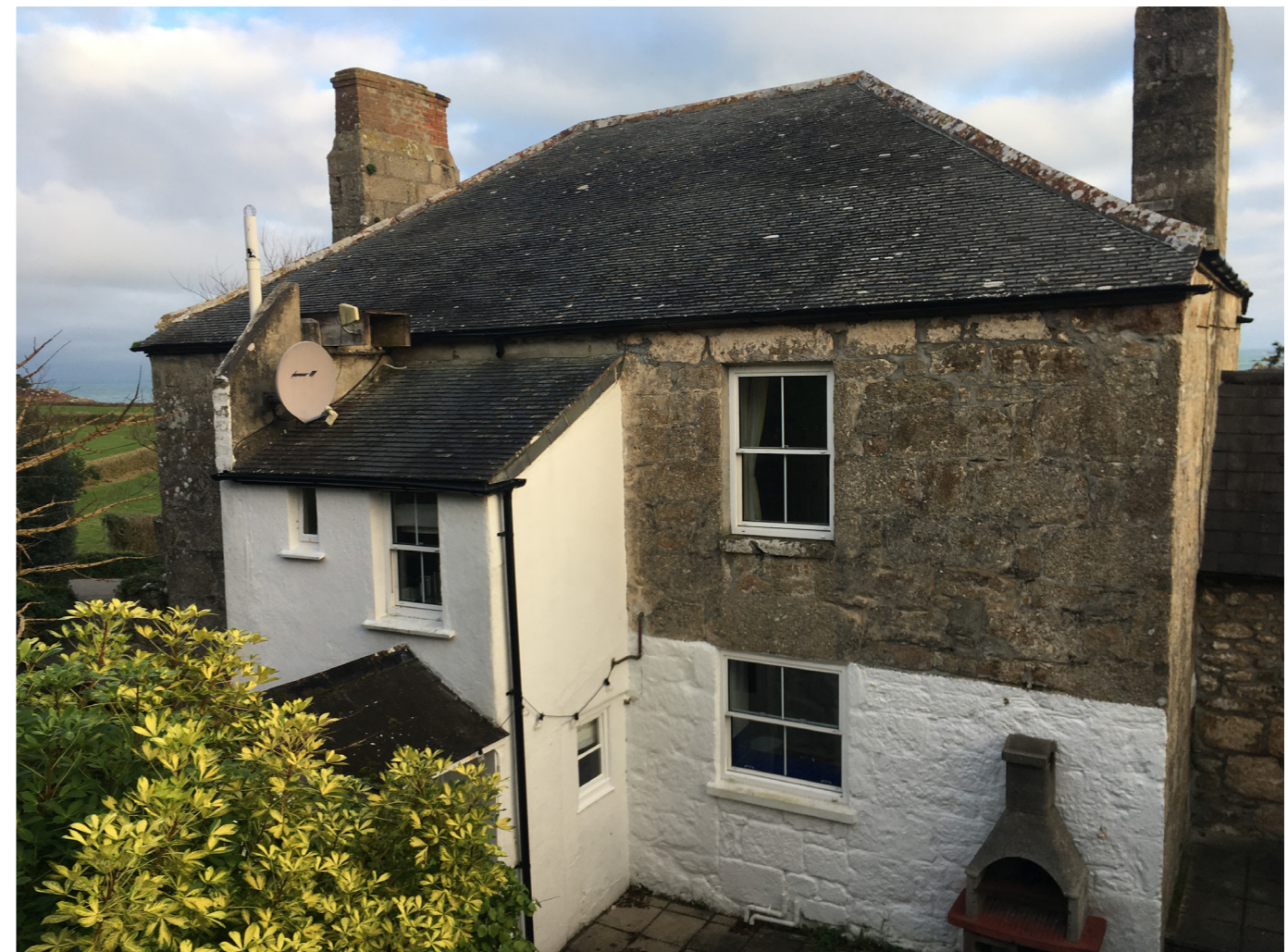
SOUTH ELEVATION - Note; blocked in door, uPVC windows & later masonry on rear face east wing.
