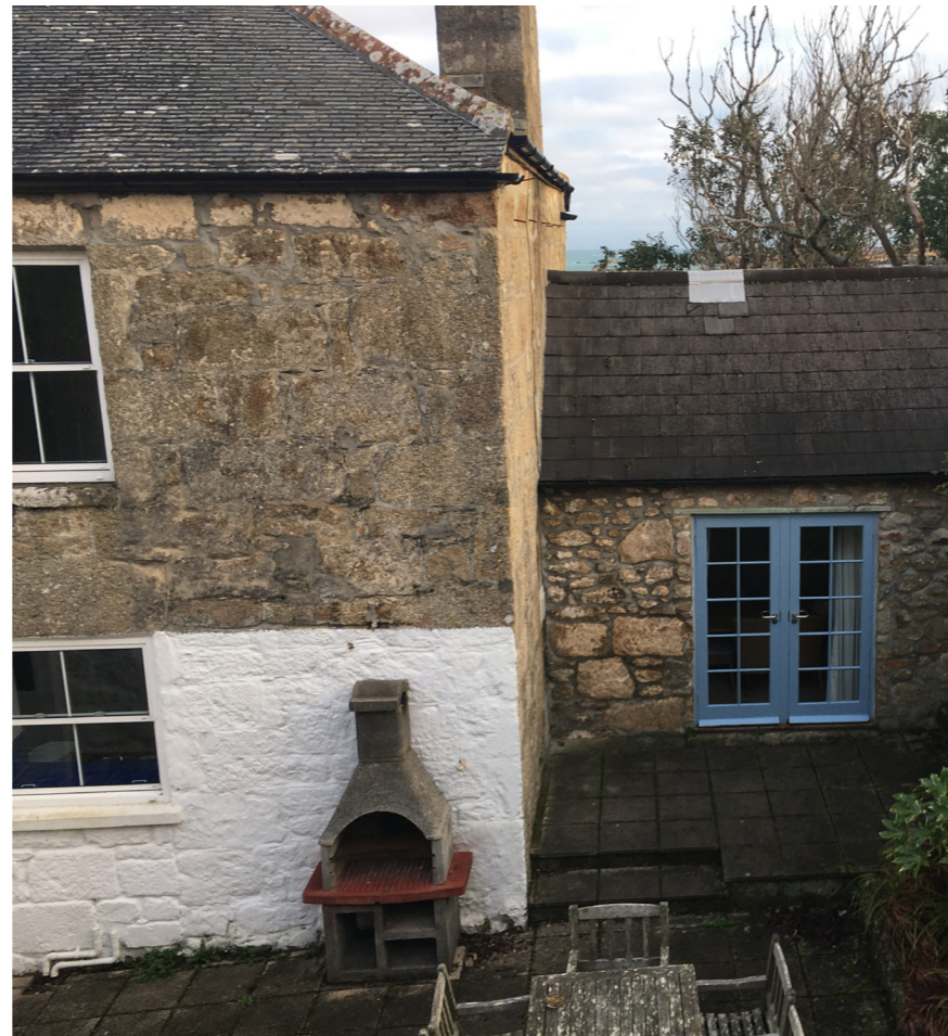
Part Rear Elevation. Note; Later granite masonry to the rear of the eastern wing (uncoursed with Grey cement pointing); GLF rear window is an infilled door.
