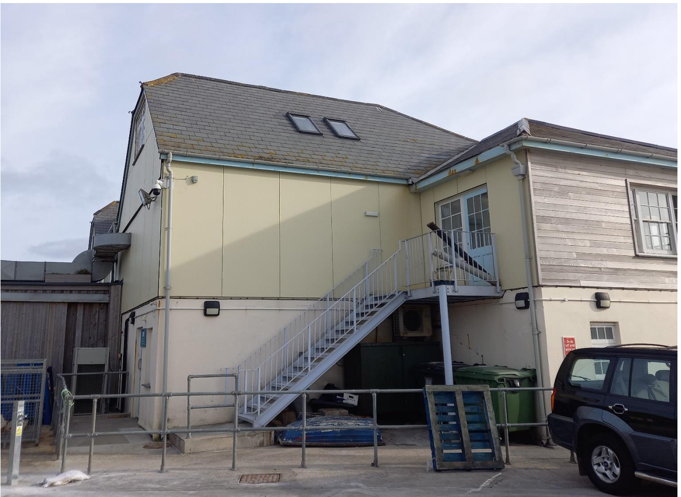
Photo 2. – showing velux (right side) which will be moved and the numerous security lights
