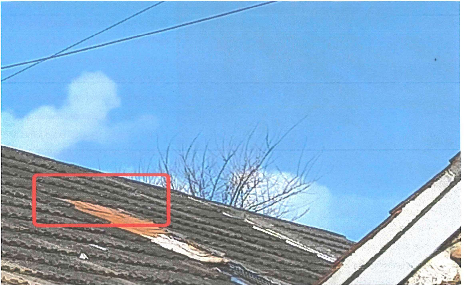
Photo 2. Gap between underlying sarking and roof tiles
