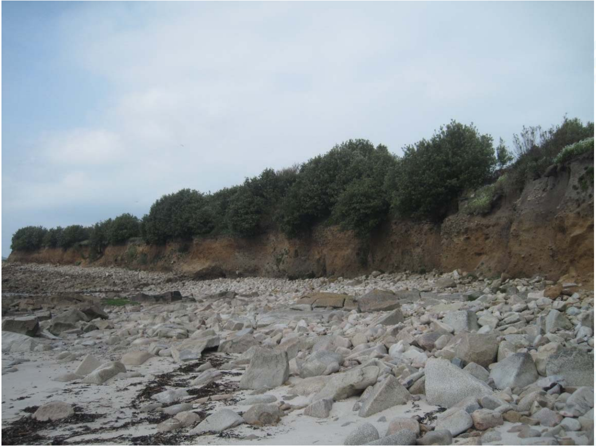
Figure 4-15: Erosion of ram cliff in northern part of bay
