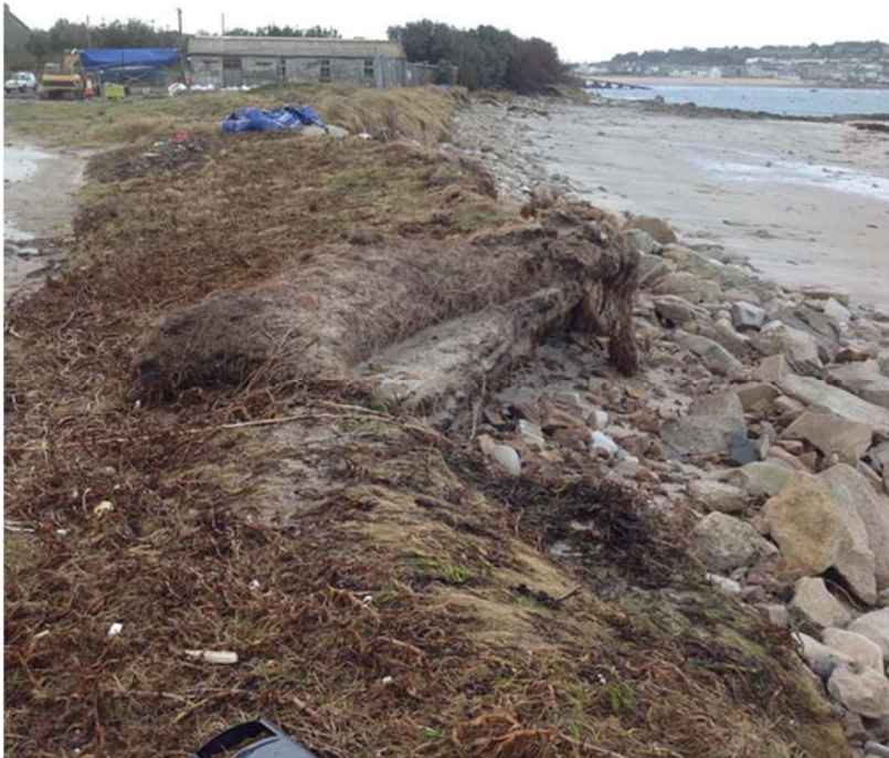
Figure 4-29: Erosion of bank after 2014 storm
