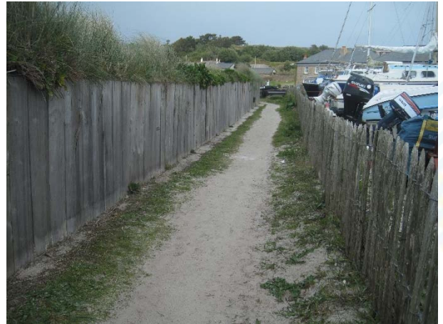
Plate 4: Rear of dune stabilisation works adjacent to the boat yard showing greenheart timber clad retaining wall
