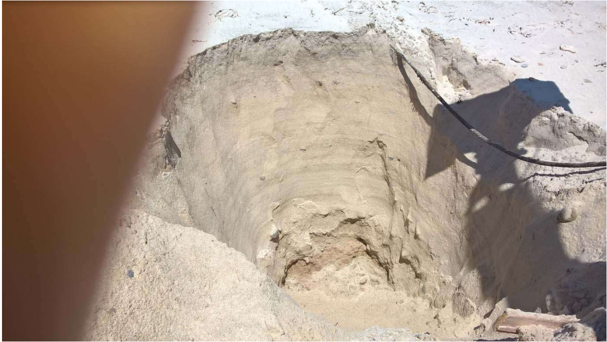
Fig 2 –Pit 1 South Beach (note; steel cable uncovered during excavation – not labelled and not marked on any maps – does not coincide with cable to BT communications supply which is some 15-20m to east of this point)
