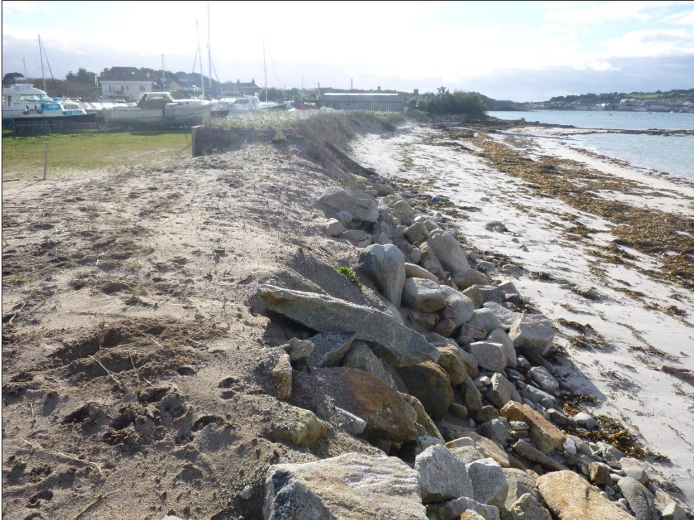
Figure 4: Looking south at the midpoint of the beach showing the interface between the existing dune defence in the background and the ad-hoc revetment in the foreground.
