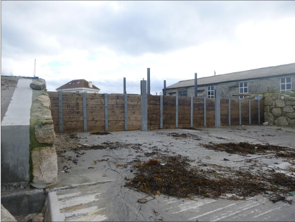
Figure 6: Boatyard slipway protected by stop-logs at the southern end of the beach. Logs branded with D of C (Duchy of Cornwall) who are believed to be responsible for slipway and existing dune defence.
