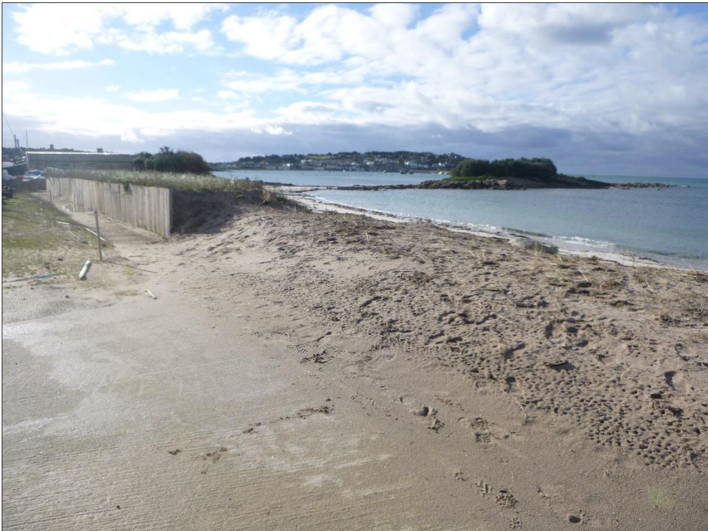
Figure 5: View of the existing dune defence and its timber sleeper construction. Note the low spot of the existing bank in the foreground that was formerly used as a temporary beach access point during the St. Mary's quay extension works in 2014/15.
