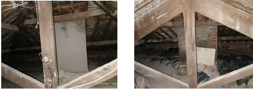
Photos 5 and 6. Showing the interior of the roof void over the house
