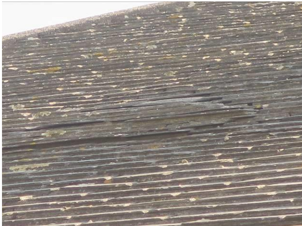
Photograph 3: Showing the area of the roof where the tiles have slipped.
