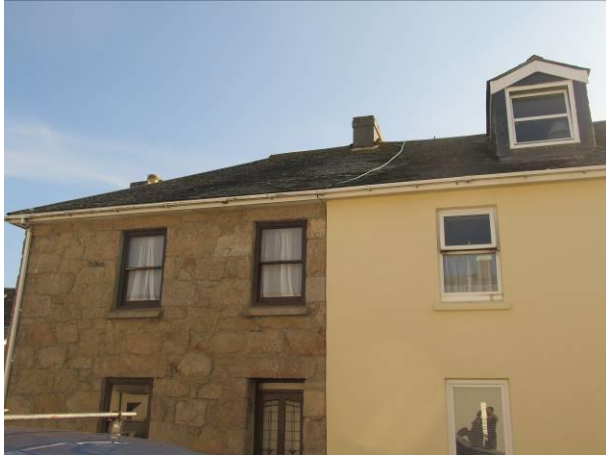
Photograph 1: Showing the western aspect of 1 and 2 Buzza Street. The granite blockwork of 1 Buzza Street and the rendered façade of 2 Buzza Street distinguish the two properties.
