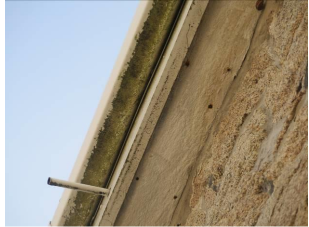
Photograph 2: Showing the underside of the boxed eaves illustrating the tight fitting and lack of access. The guttering attached to a fascia board can be seen to the left.
