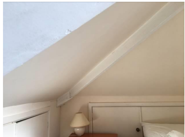
Photograph 4: Showing the interior of the roof space at 1 Buzza Street where the residential conversion has occurred. The built-in storage close to eaves level can also be seen.
