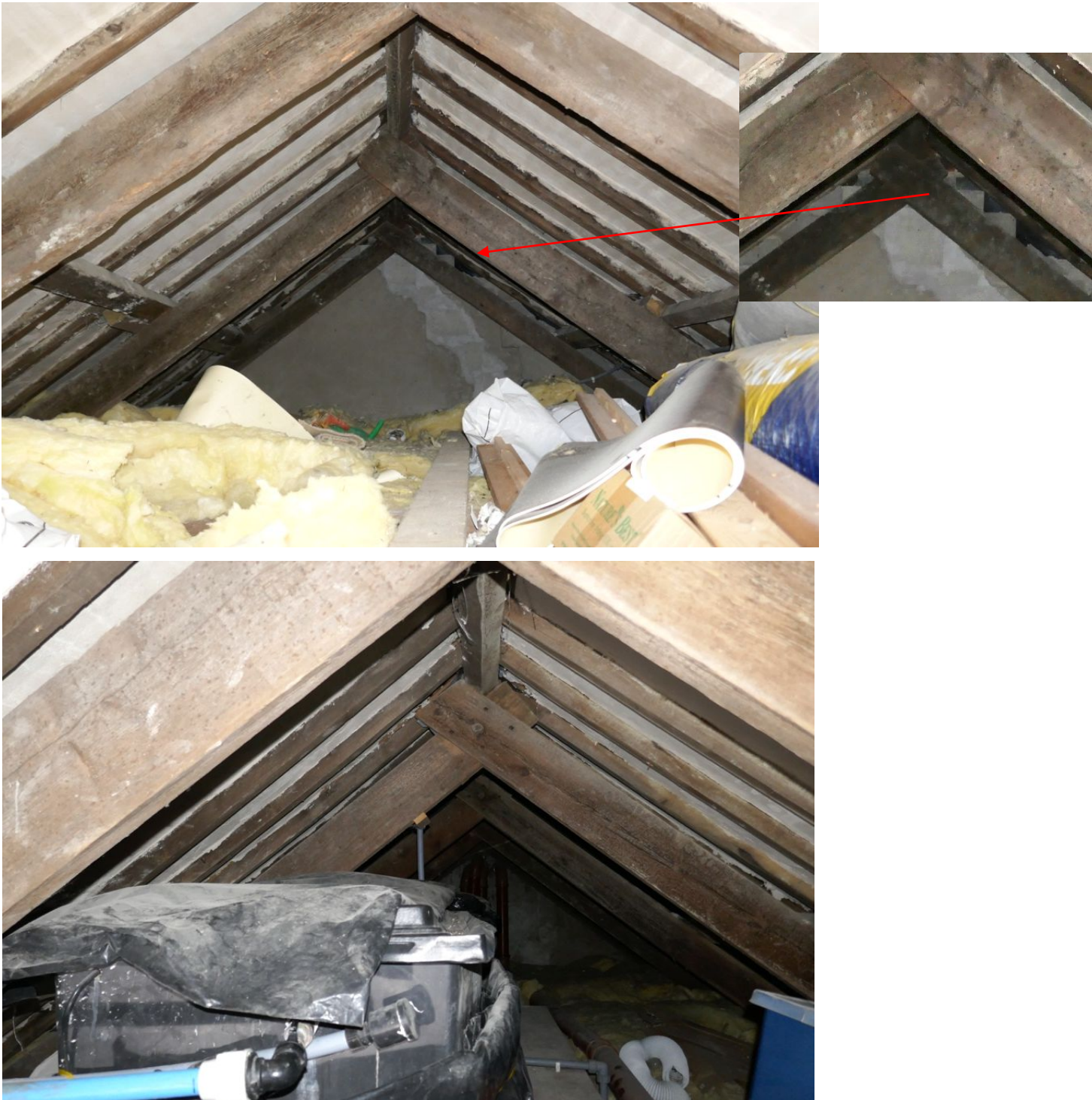
Top: Roofspace looking to the rebuilt south elevation showing incomplete infill to the west side
