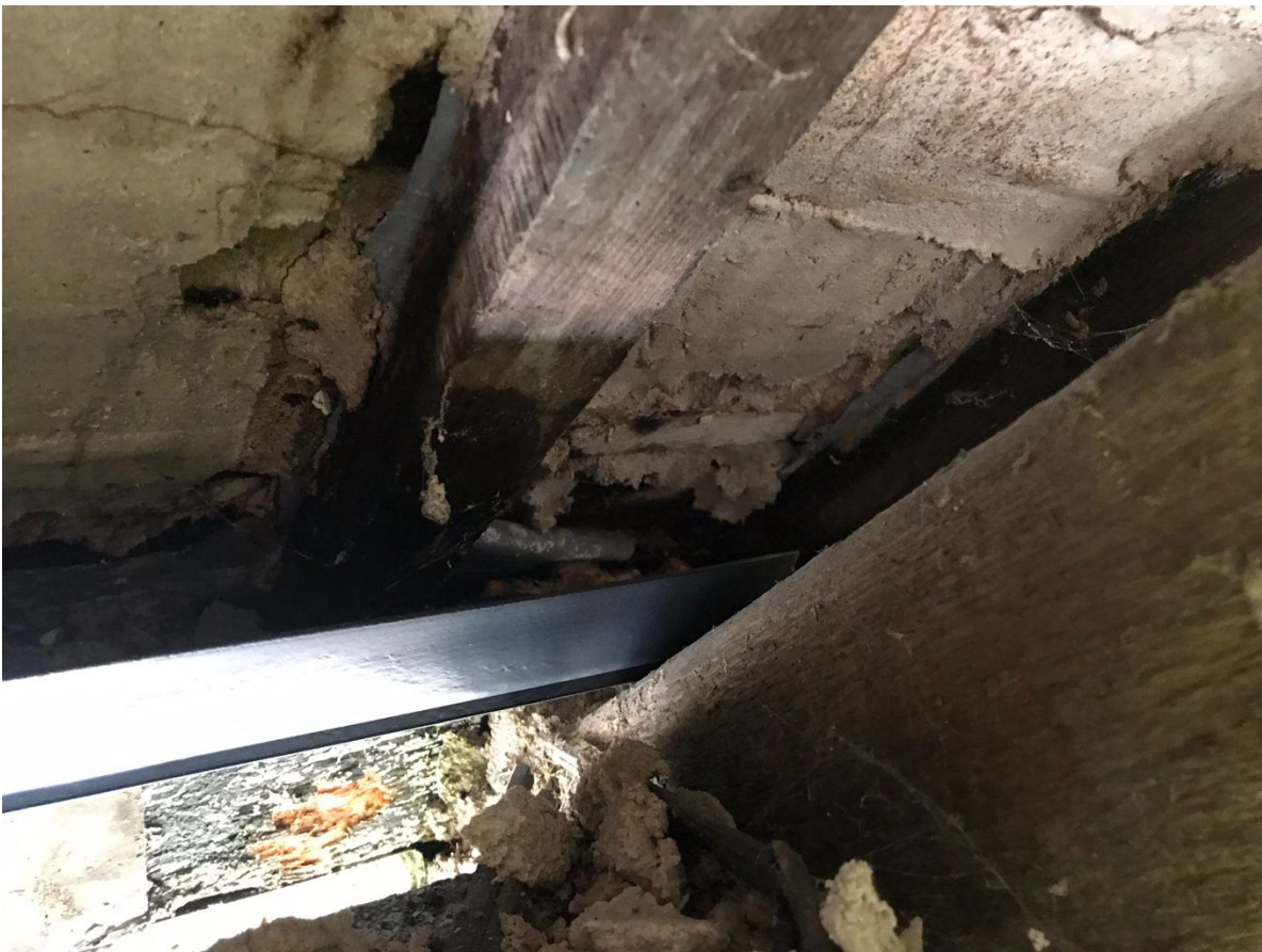
Photographs courtesy of the Duchy of Cornwall showing the temporary repair above the bathroom window to provide drainage
