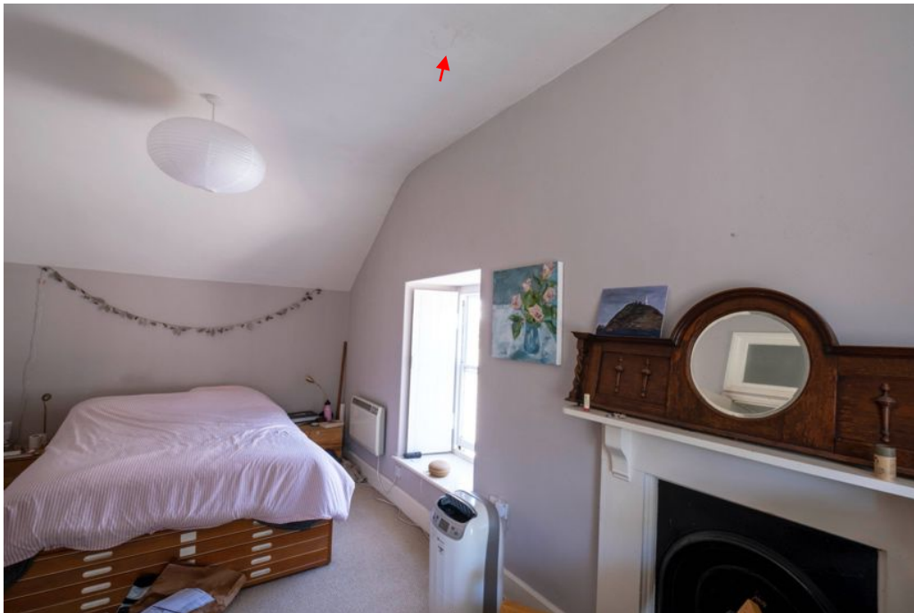
Top: South Bedroom showing damp to ceiling within 2 years of painting.
