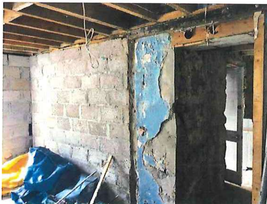
Photograph 10: Showing the interior of the garage with exposed breeze block walls and exposed timber roof structure above.
