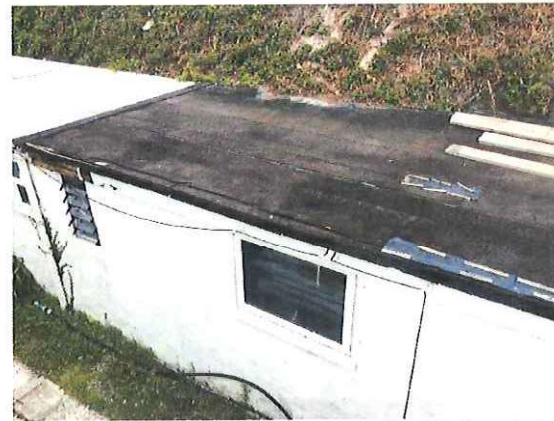
Photograph 6: Showing the exterior of the chalet building with the rendered wall, uPVC window and felted roof visible.
