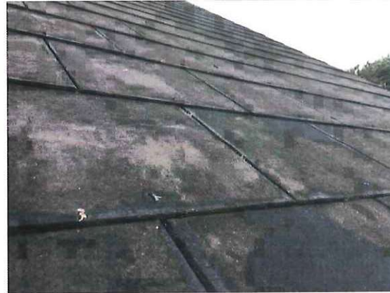
Photograph 4: Showing the tightly fitted slate roof on the existing property. This is the retained roof into which the new roof structure of the bathroom dormer will be tied.
