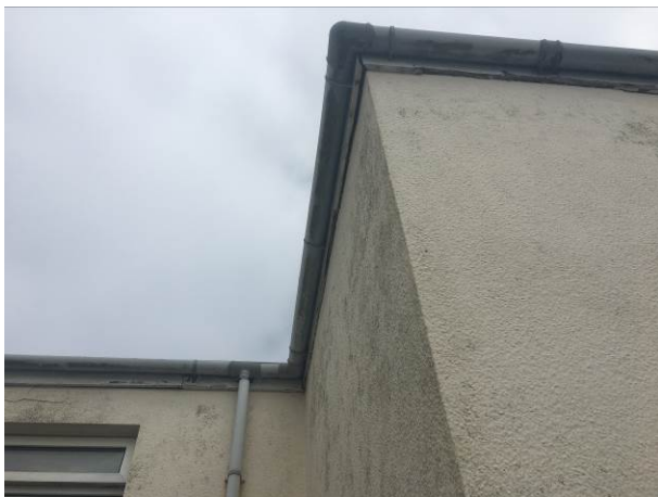
Photograph 5: Showing the fascia boards behind which gaps occur in several locations around the two-storey extension.
