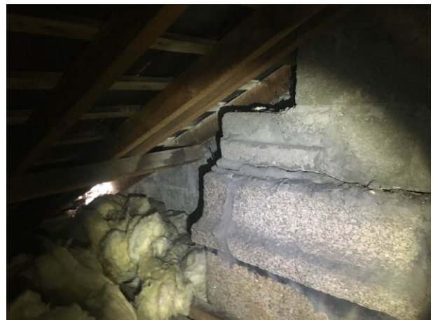
Photograph 6: Showing the granite chimney within the loft with slate tiles directly onto battens and light visible at the eaves indicating potential for internal access.
