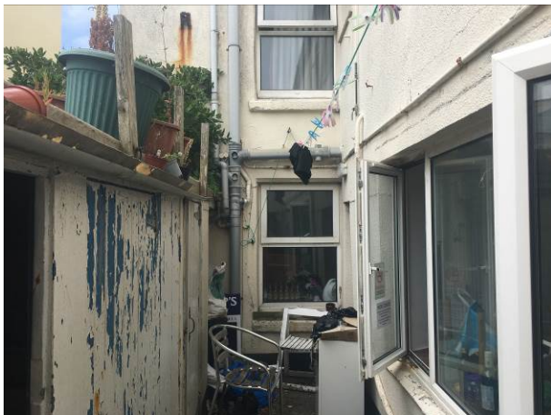
Photograph 3: Showing the alleyway on the southern aspect with the outbuildings to the left; the main 3-storey house ahead and centre; and the 2-storey flat-roof extension on the right.
