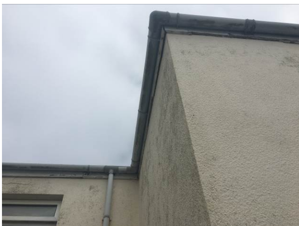
Photograph 5: Showing the fascia boards behind which gaps occur in several locations around the two-storey extension.
