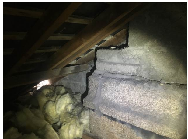
Photograph 6: Showing the granite chimney within the loft with slate tiles directly onto battens and light visible at the eaves indicating potential for internal access.
