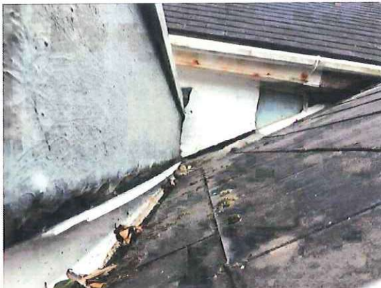
Photograph 3: Showing the existing gully between the fibre-glassed back wall of the dormer and the slate roof of the main property
