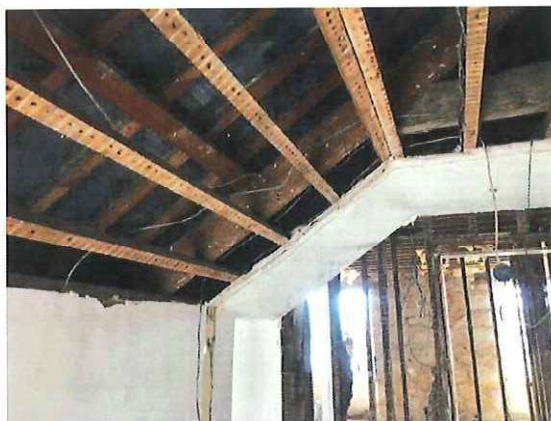
Photograph 5: Showing the interior of the roof of the main residential dwelling. This is the roof into which the new roof structure of the replacement bathroom dormer will be tied.
