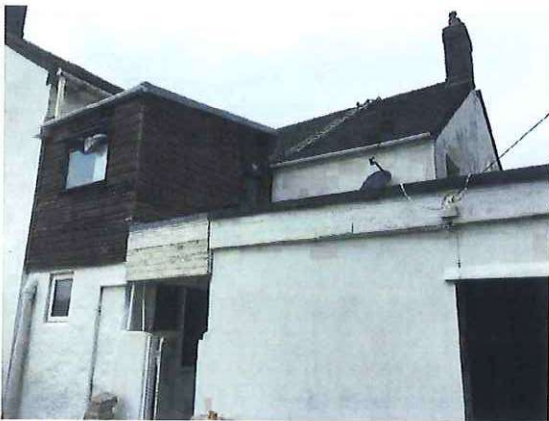
Photograph 9: Showing the garage (bottom right) with the open door visible. The bathroom dormer can be seen to the upper left of the image.
