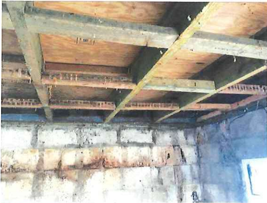
Photograph 7: Showing the interior of the chalet with exposed timber framework and chipboard above. The exposed breezeblock walls can also be seen.
