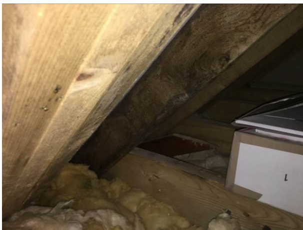
Photograph 5: Showing the interior of the eaves loft space where the new roof of the extension will tie in.
