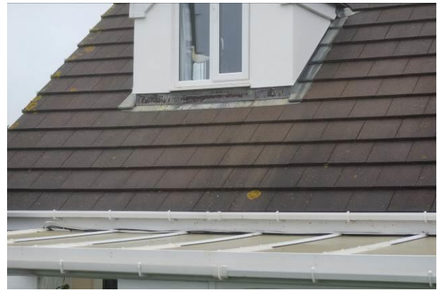
Photograph 4: Showing the pitch of the roof where the new extension roof will tie in – the interlocking concrete tiles are well fitted and in excellent condition.
