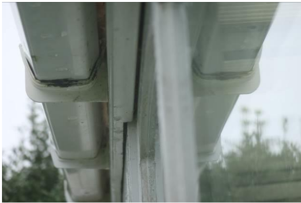
Photograph 3: Showing the gaps in the fascia above the conservatory windows – these gaps are too tight and superficial to allow access by roosting bats.
