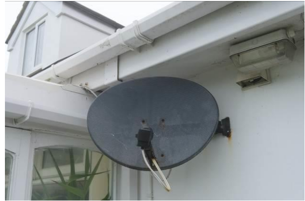
Photograph 2: Showing the union between the conservatory (left) and the main dwelling with the well-fitted uPVC boxed soffits visible.
