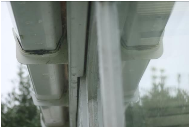
Photograph 3: Showing the gaps in the fascia above the conservatory windows – these gaps are too tight and superficial to allow access by roosting bats.
