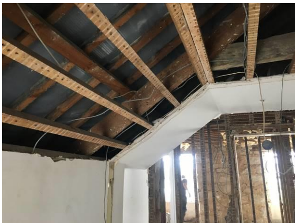
Photograph 5: Showing the interior of the roof of the main residential dwelling. This is the roof into which the new roof structure of the replacement bathroom dormer will be tied.
