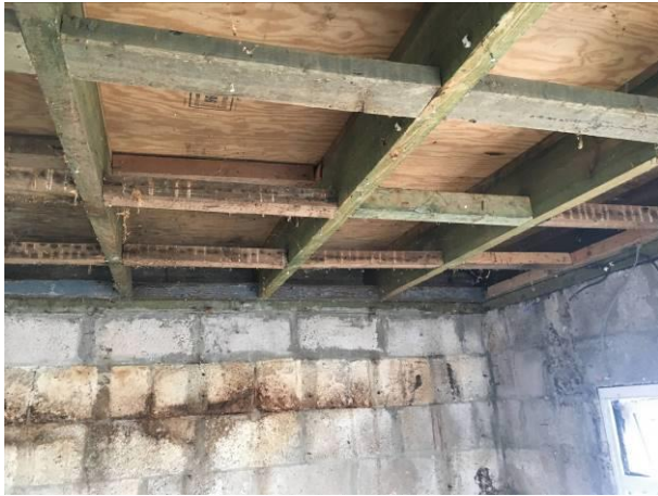
Photograph 7: Showing the interior of the chalet with exposed timber framework and chipboard above. The exposed breezeblock walls can also be seen.
