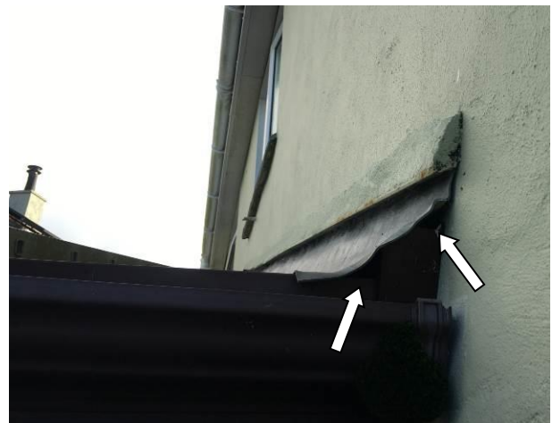
Photograph 6: Showing the lead flashing at the joint between the conservatory roof to the adjacent building – there are minor gaps present where indicated.
