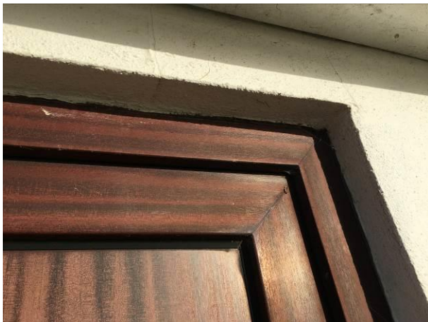
Photograph 3: Showing well-fitted uPVC door frame – this is illustrative of the condition of window and door frames associated with the property.
