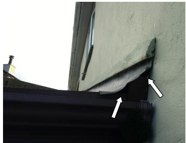
Photograph 6: Showing the lead flashing at the joint between the conservatory roof to the adjacent building – there are minor gaps present where indicated.
