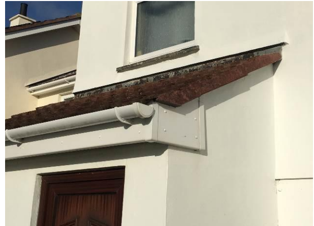
Photograph 2: Showing a closer view of the porch roof with the well-sealed uPVC soffit on the front, and the well-sealed verge on the gable.
