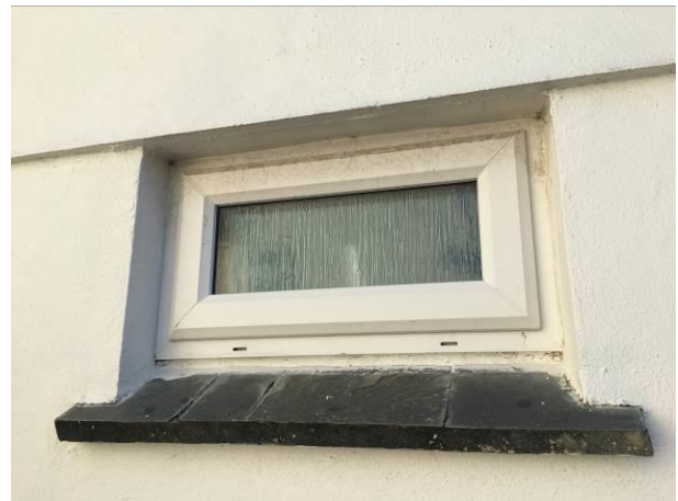
Photograph 4: Showing the porch window – the uPVC frame is well-fitted and the slate sill is well sealed.
