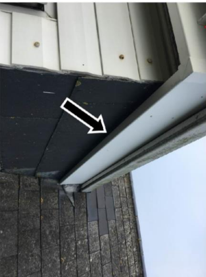
Feature C - Minor gap behind fascia above hanging tiles on dormer (north and south aspects)
