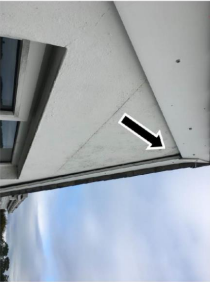
Feature B - Minor gap behind fascia on east-facing gable.
