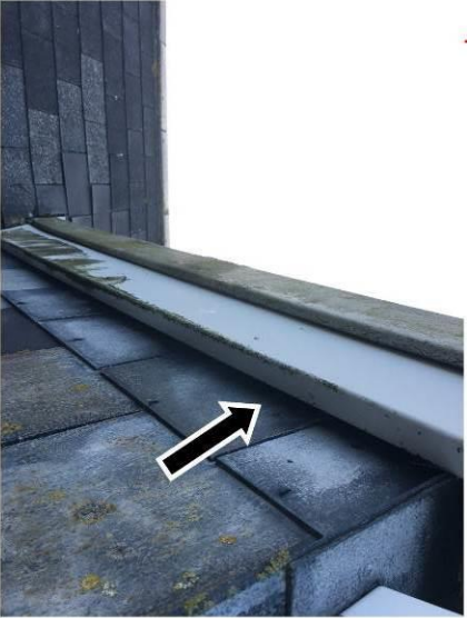
Feature D - Minor gap behind fascia above hanging tiles on dormer (north and south aspects)
