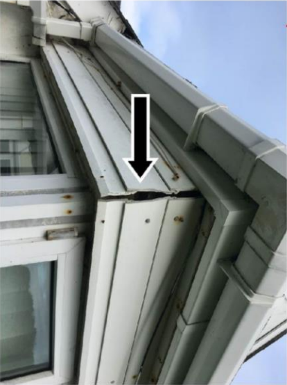
Feature A - Gaps behind fascia on south-eastern corner of flat roof section
