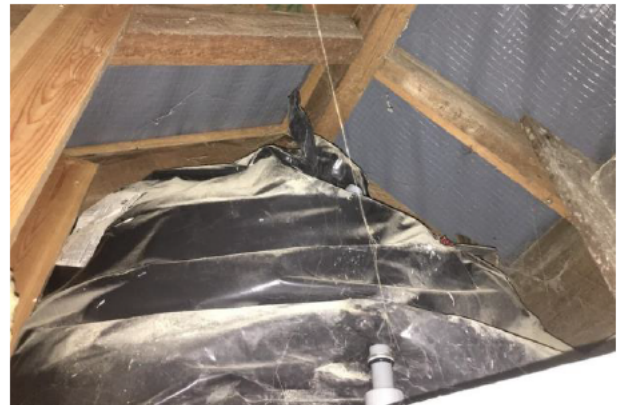
Photograph 4: Showing the accessible loft space with water tank. The new roofing membrane above the timber roof structure is visible.
