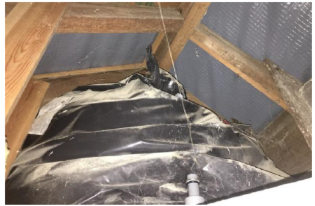
Photograph 4: Showing the accessible loft space with water tank. The new roofing membrane above the timber roof structure is visible.
