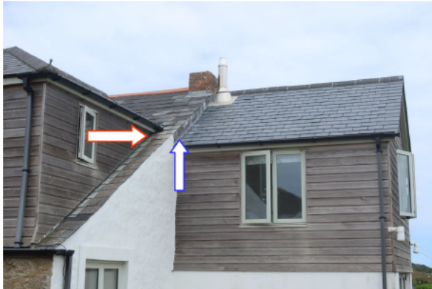
Photograph 1: Showing the brick-built chimney viewed from the west. The chimney is visible along with the change in ridge height. Examples of 'adjacent feature' locations are highlighted including the potential access to the soffit (red arrow) and lifted lead flashing (blue arrow).
