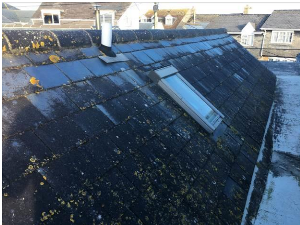
Photograph 3: Showing well-fitted roof and ridge tiles of the single-storey pitched roof component. The skylight window can be seen along with the flat roof which connects this component of the structure with the two-storey pitched roof to the east.
