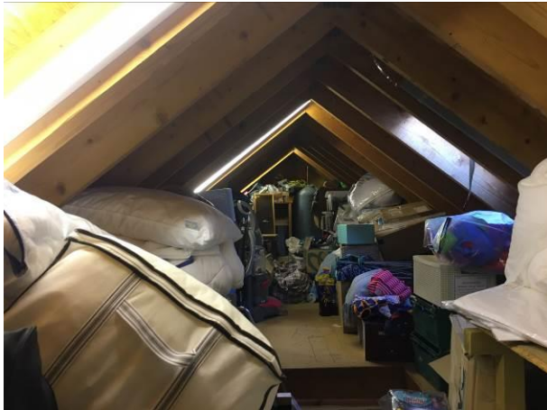
Photograph 1: Showing the interior loft space of the single-storey pitched roof component of the building.
