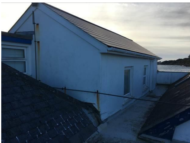
Photograph 5: Showing the two-storey pitched roof section of the building which lies to the east of the single-storey pitched roof.
