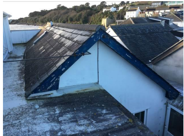
Photograph 4: Showing the northern gable of the single-storey pitched roof component of the building.
