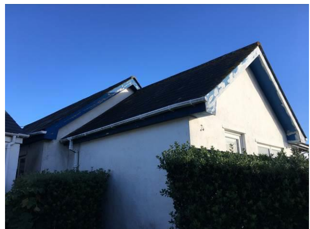
Photograph 6: Showing the southern gable and western aspect of the single-storey pitched roof section of the building which looks out onto Porthcressa.
