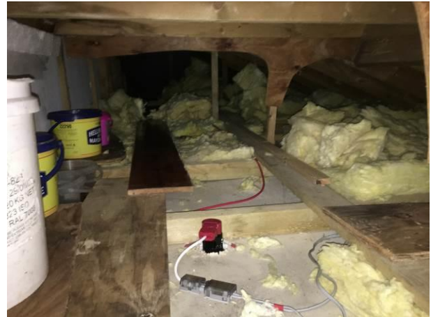
Photograph 2: Showing the interior loft space of the single-pitch roof which runs along the southern aspect of the building.
