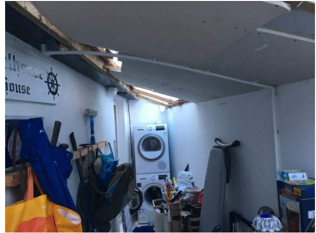
Photograph 8: Showing the inside of the lean-to building used as a utility and storage space.
