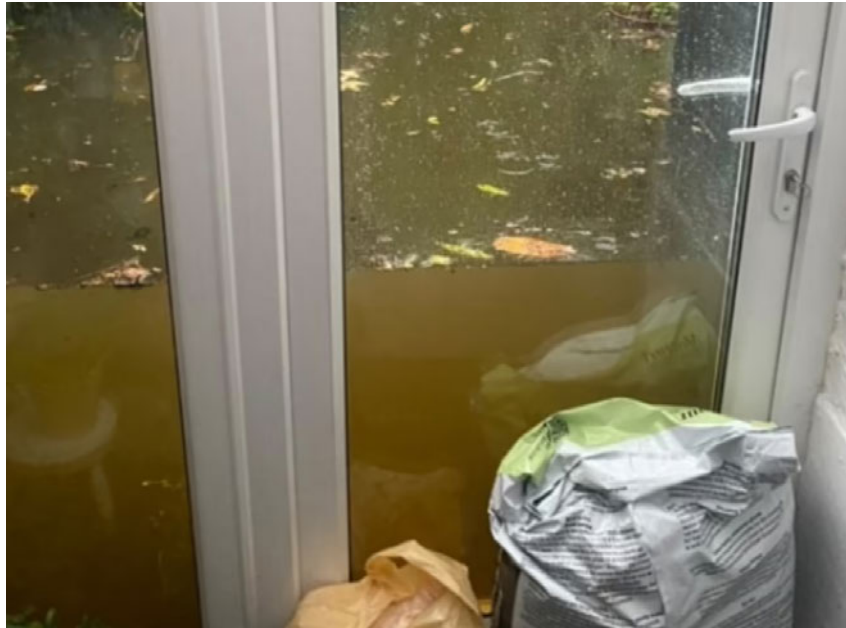
Figure 7: UPVC doors under flood conditions. These appear to offer reasonable flood resilience
