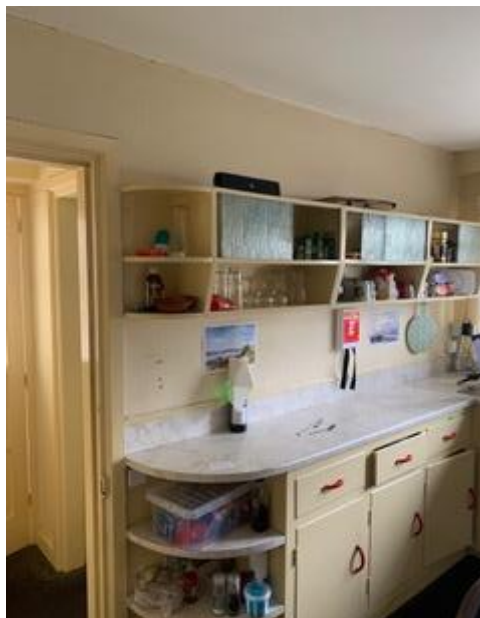
Fig. 19: The south-east wall of the existing kitchen, with doorway to the conservatory.
