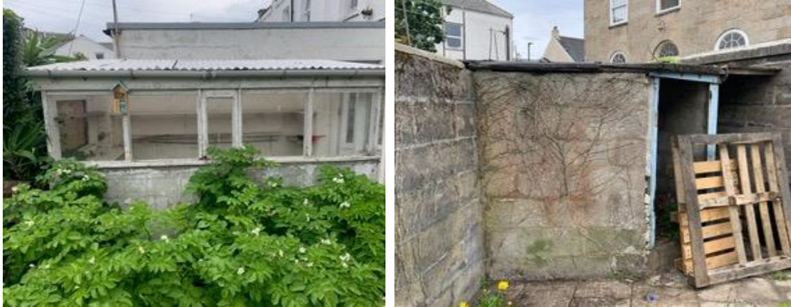
Fig. 15 A and B: The existing greenhouse (left) and coal-store (right) to the rear of the property.
