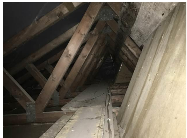
Photograph 6: Showing the loft space of the pitched roof Section B which could not be fully inspected due to the size and construction.
