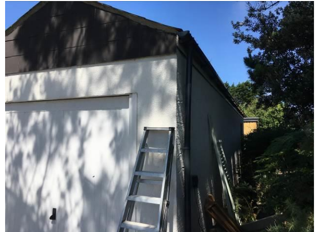
Photograph 2: Showing the property from the south-east with the pitched roof Section B over the garage unit.
