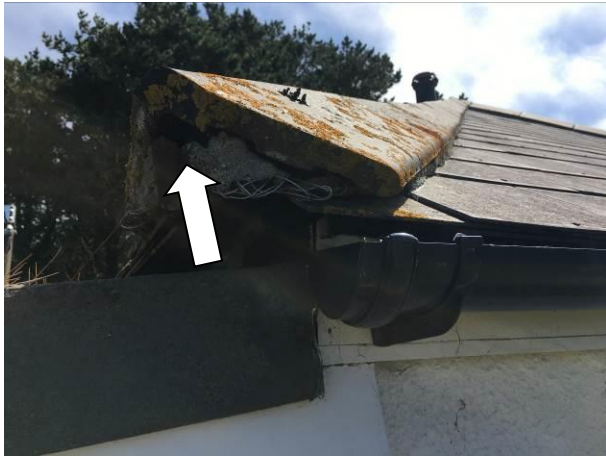
Photograph 7: Showing an example of the minor sections of missing pointing at the base of the hipped ridge tiles in roof Section A.
