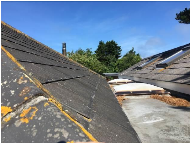
Photograph 3: Showing the flat roof Section C at the point where it links the other two roofs.
