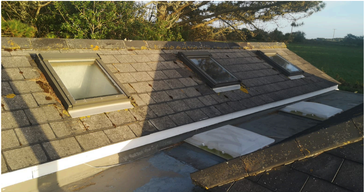
Above: The pitched roof over the garage, corner of the main hipped roof and flat roof connecting link
