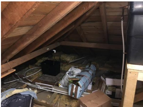
Photograph 5: Showing the interior of the loft space of the hipped roof Section A – the sarking boarding above the timber trusses can be seen.
