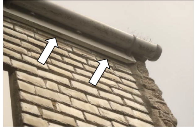
Photograph 8: Showing an example of the gaps beneath the fascias which occur around the structure. These offer potential roosting opportunities for bats in their own right, as well as access to further opportunities associated with the wall plate and slate tiles.
