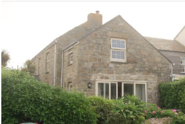
Photograph 3: Showing the extension on the western edge of the property – the second-storey room in this location is built into the rafters with no void present.
