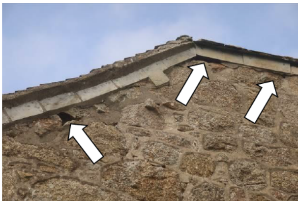
Photograph 5: Showing an example of the gaps on the north-eastern gable with confirmed nesting sparrows – these features would also allow access to potential roosting opportunities for bats.
