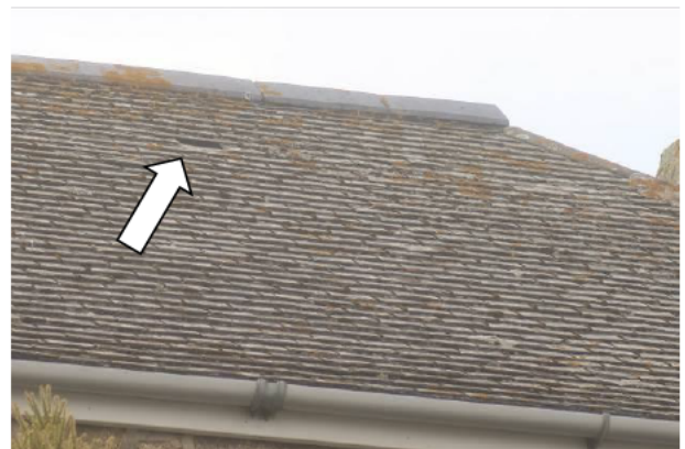
Photograph 6: Showing an example of the occasional gaps in the pointing of the tiles which could provide access or roosting opportunities for bats.
