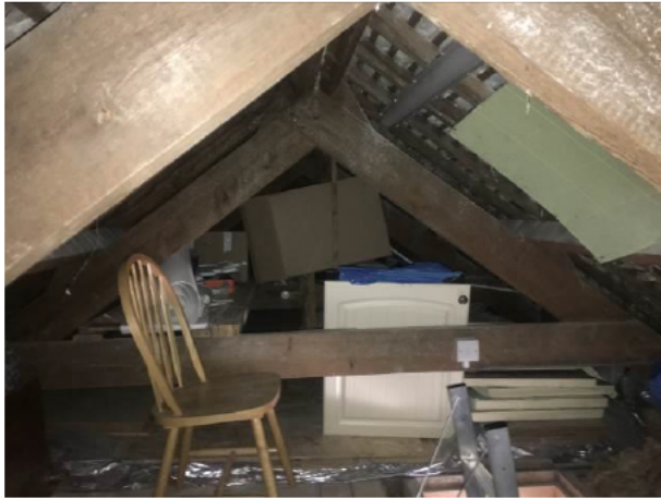
Photograph 7: Showing the interior of the loft space built around a timber truss framework.. The use of the space for storage, restricting comprehensive inspection, can be seen.
