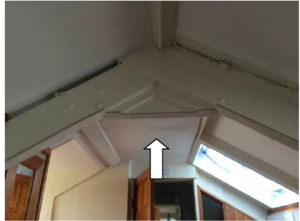
Photograph 2: Showing the top floor of the property with some minor apex voids (as indicated) but with the ceiling built to the ridge beam in others.
