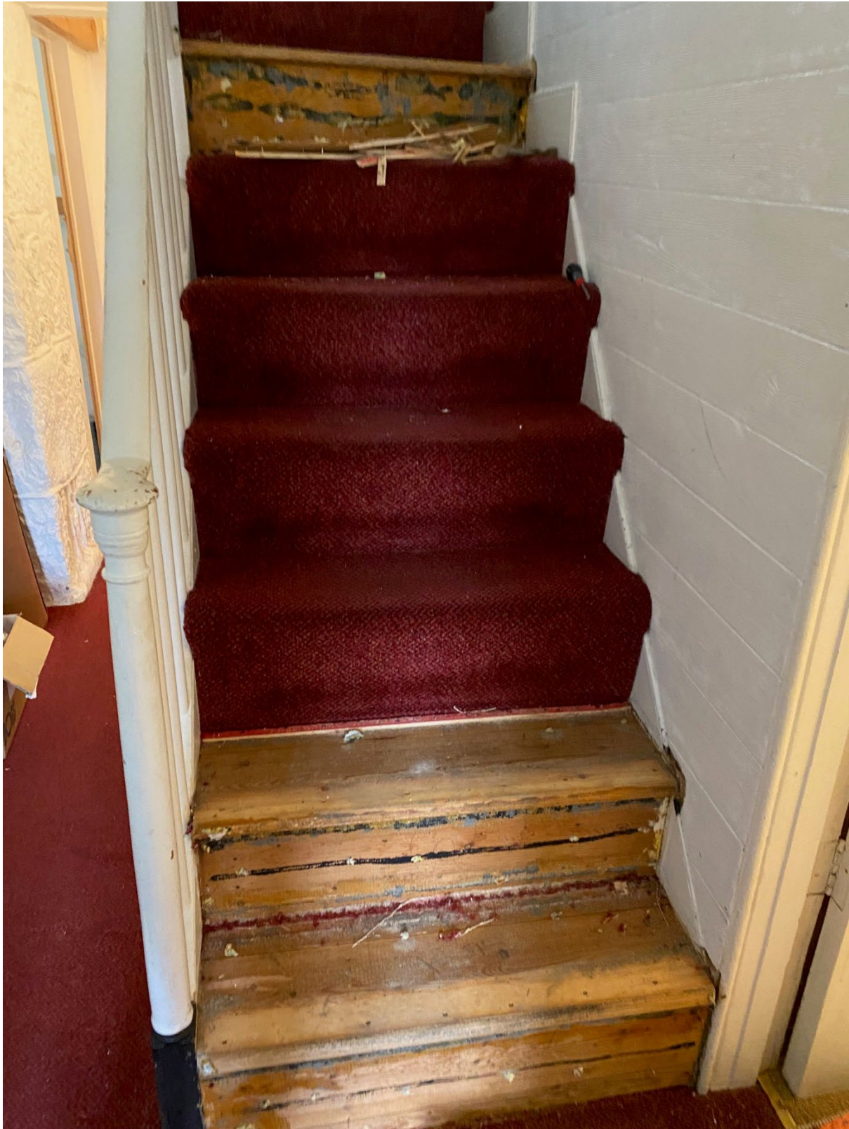
No1. This picture shows how the treads and risers have been re-fabricated and nailed together using modern round head nails to secured the treads and risers to a softwood sub frame underneath. Note how the treads come past the side strings as opposed to being housed into the string.
