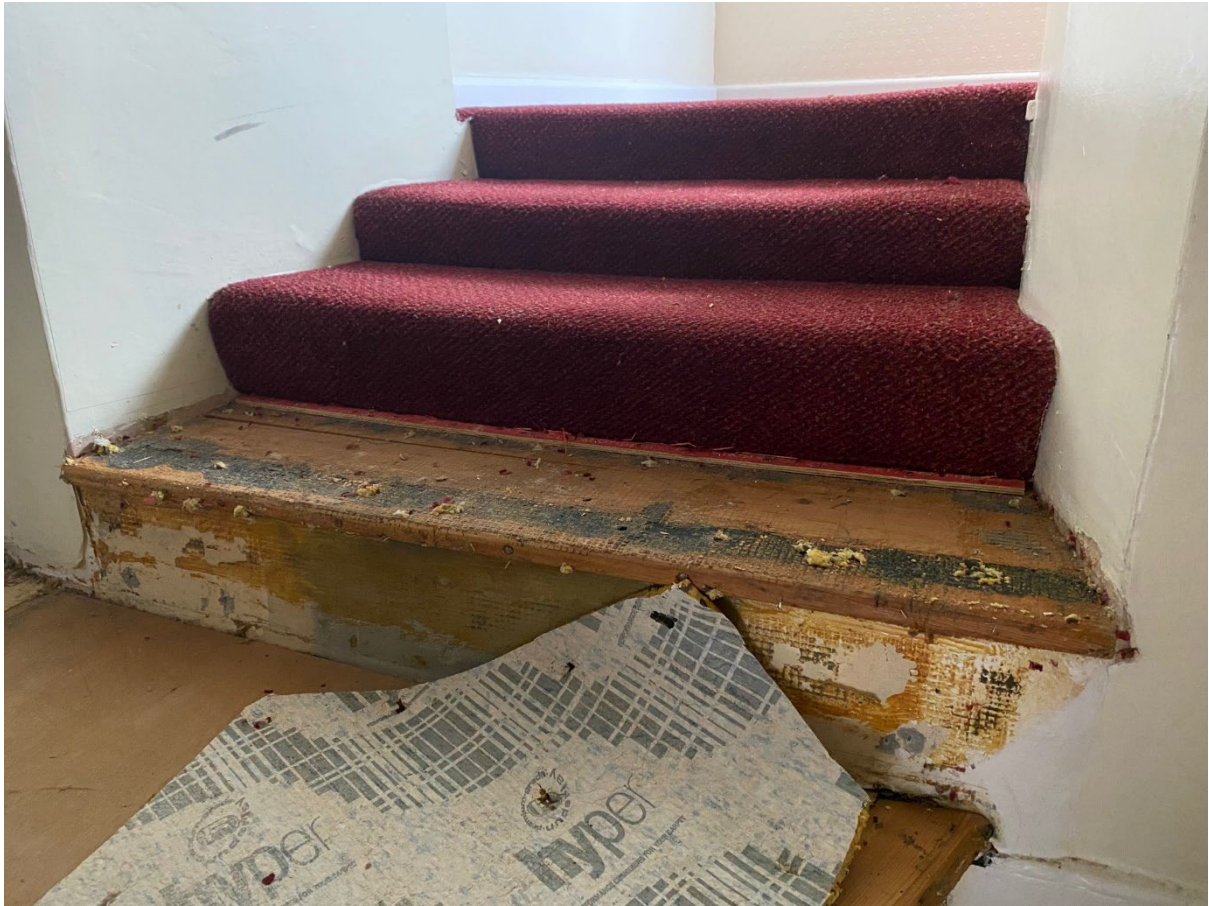
No14 Steps to rear extension showing the irregular risers and plywood to the landing.
