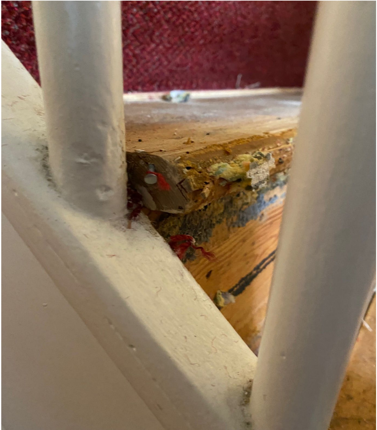
No12 Tread protruding past the string and modern balustrades
