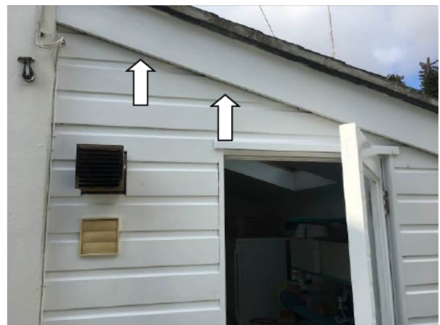
Photograph 6: Showing the access door in the lean-to component – the fascia above is indicated.
