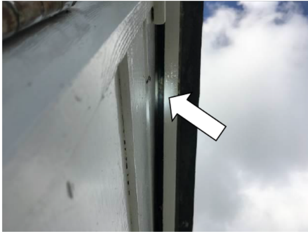
Photograph 7: Showing an example of the gaps behind the fascia on the southern aspect of the flat-roof component.
